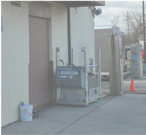
Figure 4: Existing Lift for ADA Access
