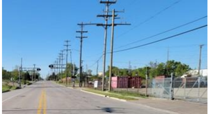
Figure 10: Overhead Lines Along 16 th St.
