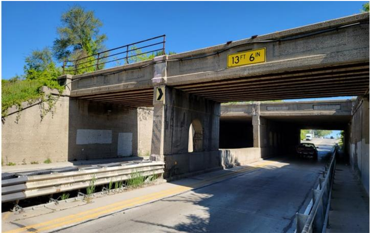
Figure 27: Existing CSXT RR Bridge over 24 th Street Bridge (CN RR Bridge in Background)
